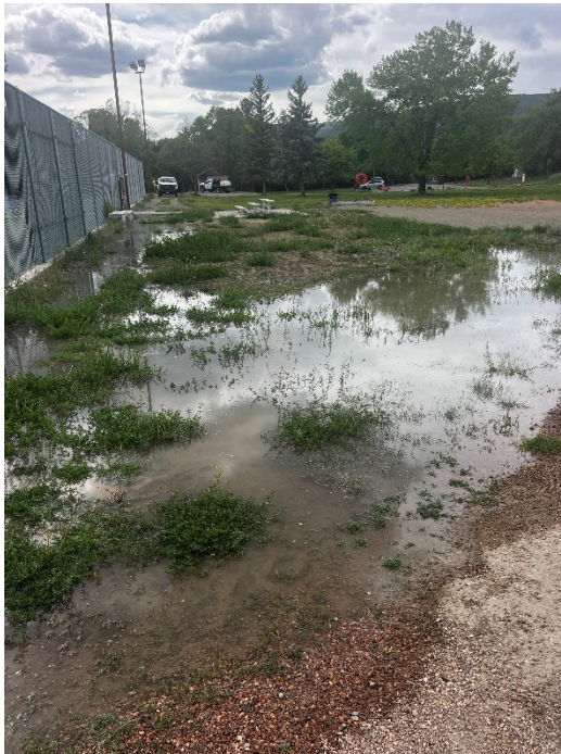
Park Sprinkler struggles- pump, and broken lines
