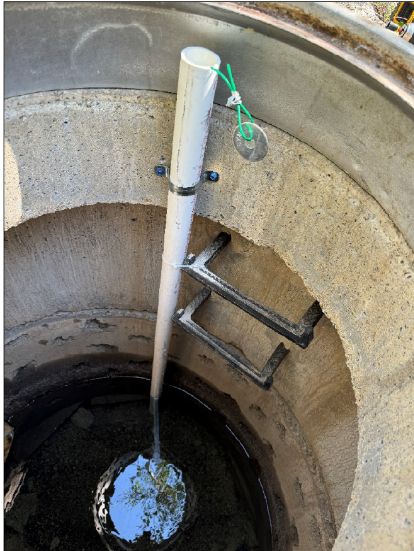
Figure 6. Installation of pressure transducer at Lake Fork Spring Box.
