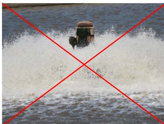
Motor is exposed to aerator spray and biomass build-up.
